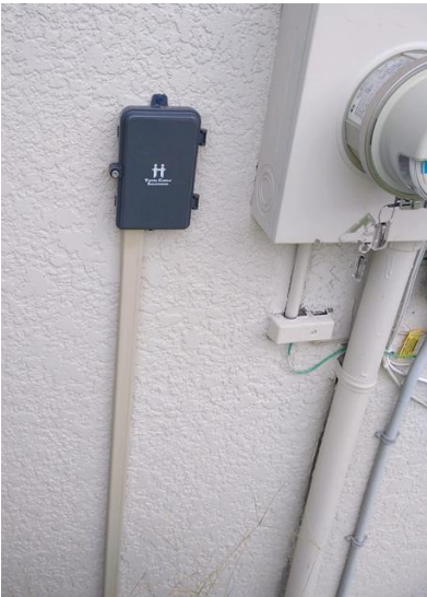
Conduit and premise box installed on home
