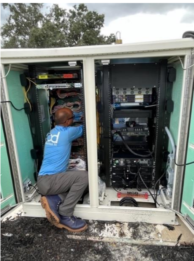
Fiber being connected in head-end cabinet
